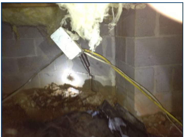
This junction box is not properly secured. The cables were on the ground
