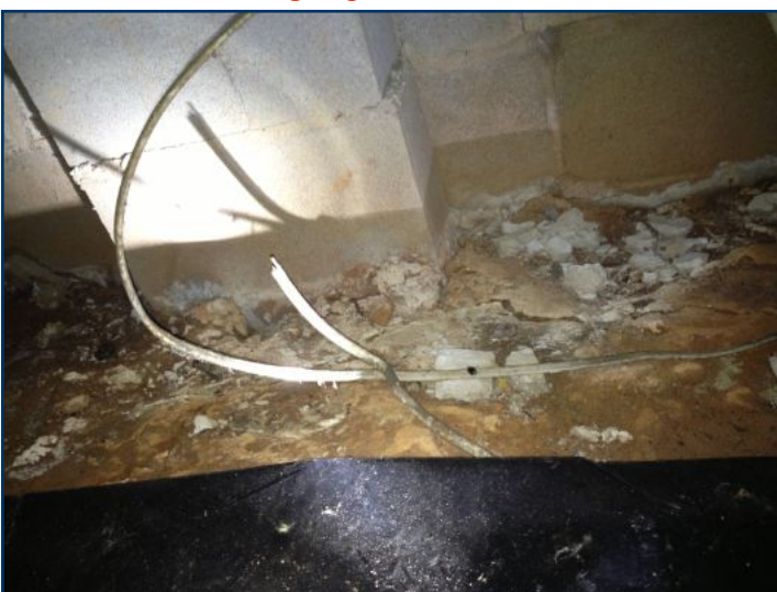
This romex cable should terminate properly in a box, or be removed.
