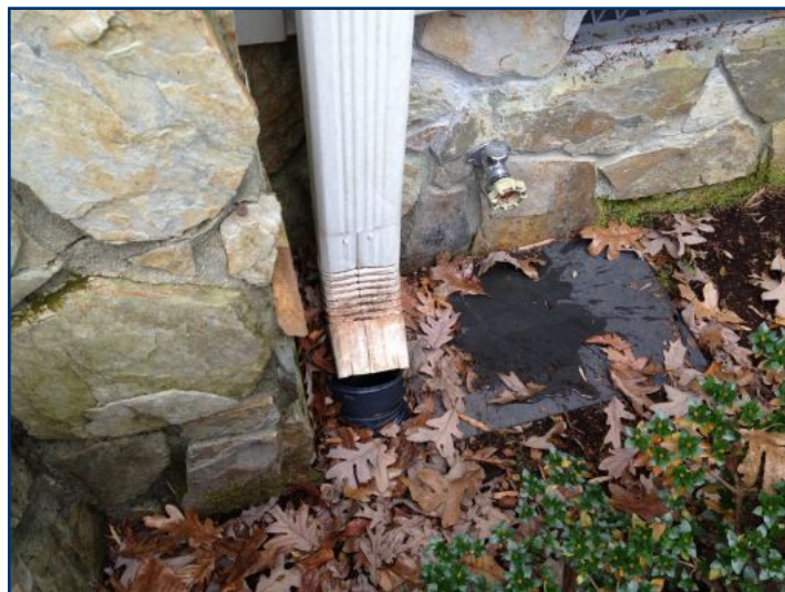
You should get the down spouts to terminate in the drainage tubes
