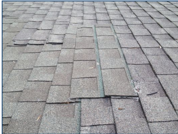
Notice the poor installation of shingles
