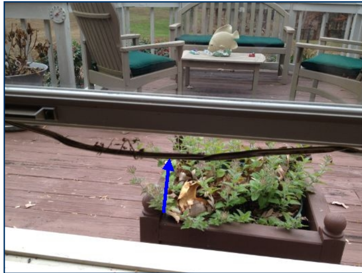
Disbonding seal on dining room window
