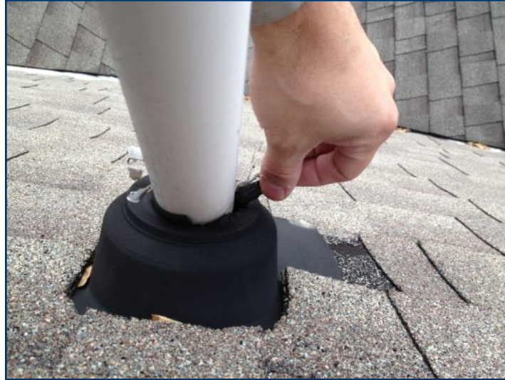
Torn plumbing vent seal
