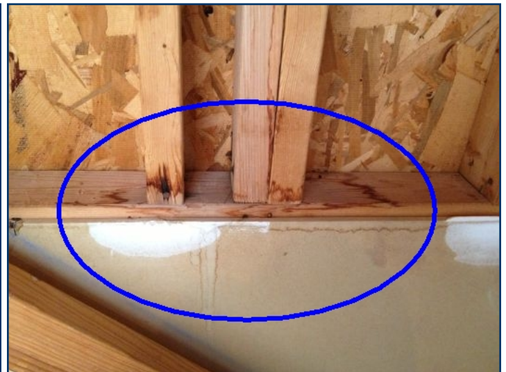
Moisture staining from gap in window
