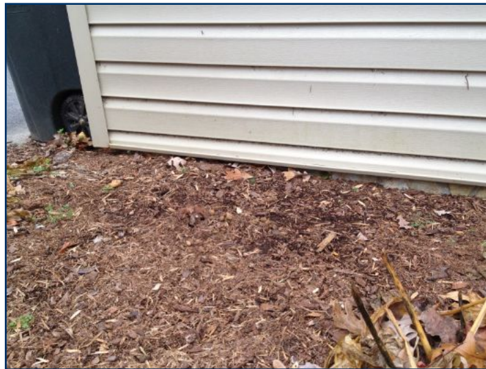
Siding in contact with the grading
