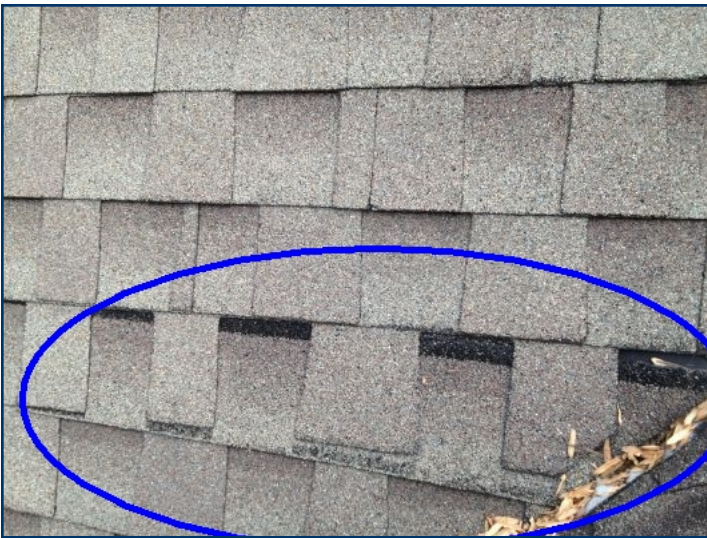
Poorly installed shingle
