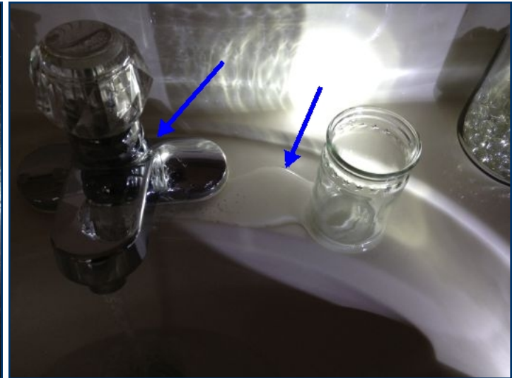
Leaking faucet in master bathroom
